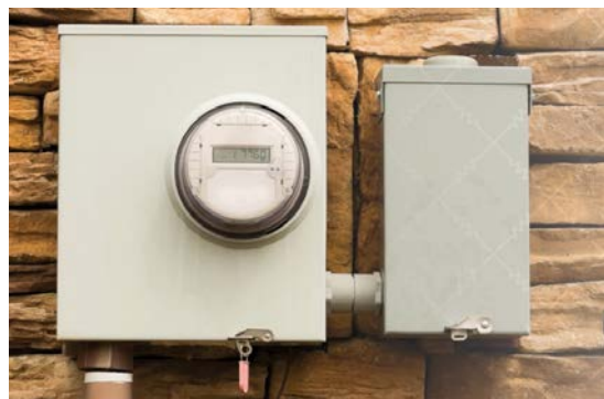
An advanced meter is installed at a home. Source. U.S. DOE. AMI and Customer Systems.
